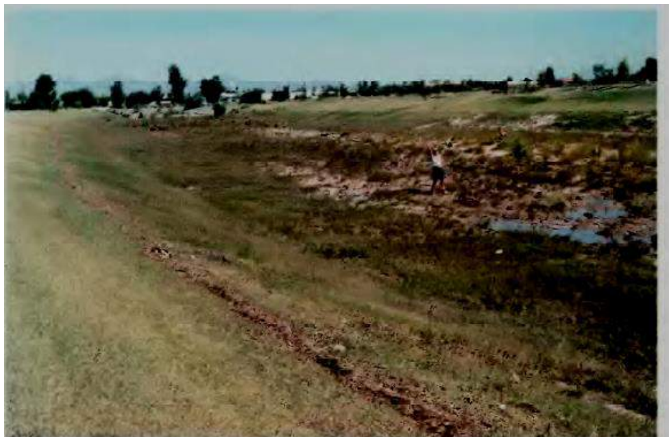
Figure 10E. View from midreach looking upstream following flow of October 6, 1993, Indian Bend Wash above Curry Road.
